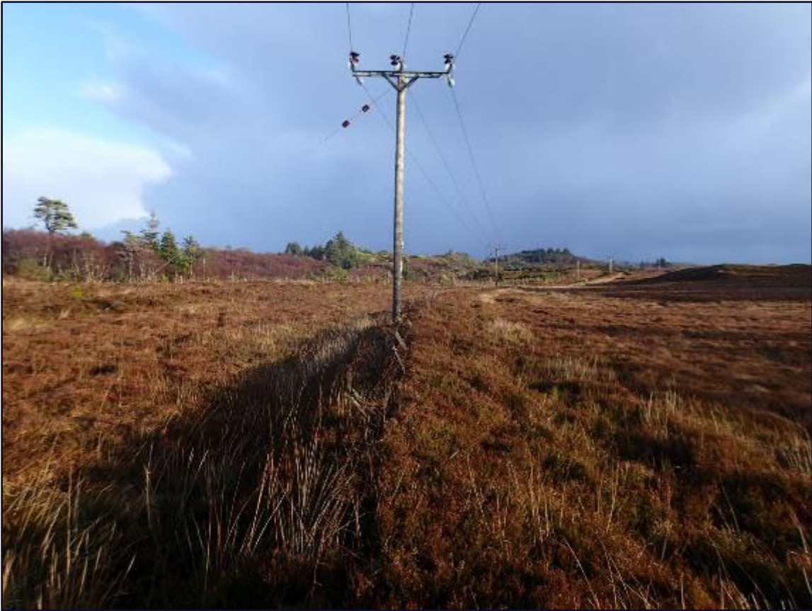
Figure 18: The "old fence" as it heads east toward the Creed. Note how the powerlines use it as a base.
