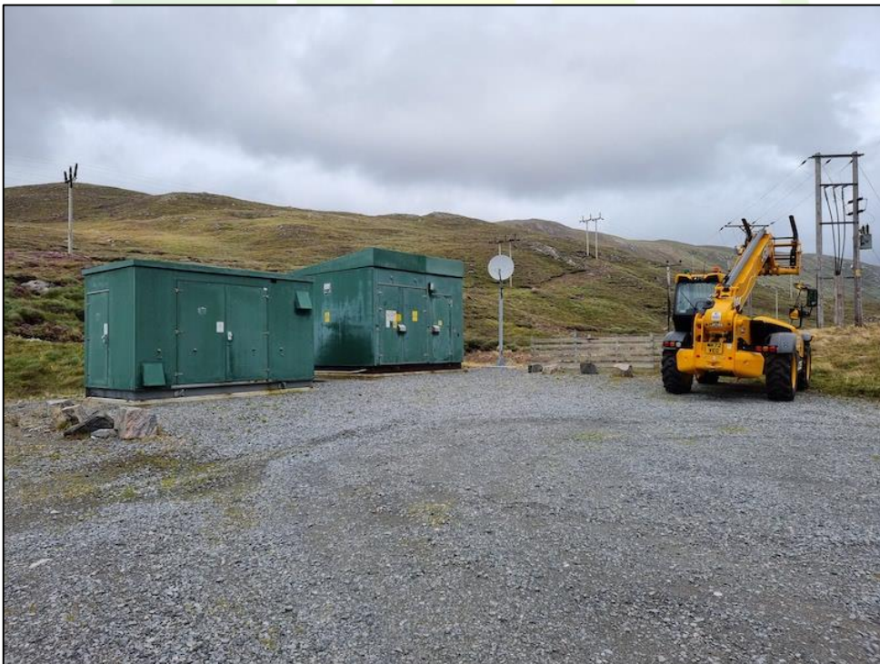
Figure 6: An area of hardstanding that sites the sub-station electrical units and machinery.
