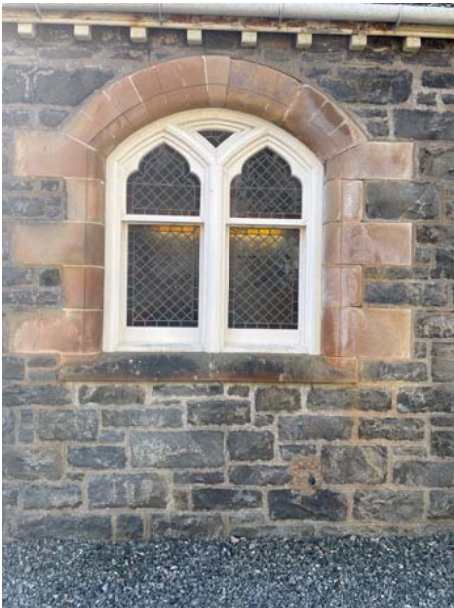
Photo 1. Existing window in east elevation to be Removed and opening extended to ground level To allow a new external entrance door to be Installed. The design of the upper part of the Window is to be retained for the screen above the Proposed new door.
