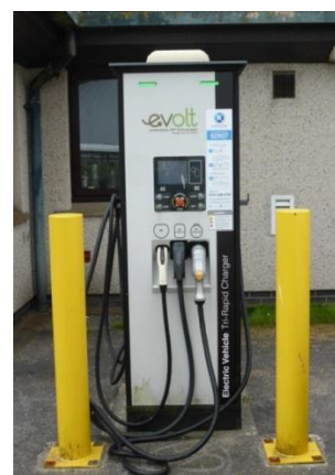
Figure 19 EV charging point
