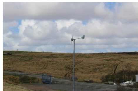
Figure 2 Evance turbine and housing site.
