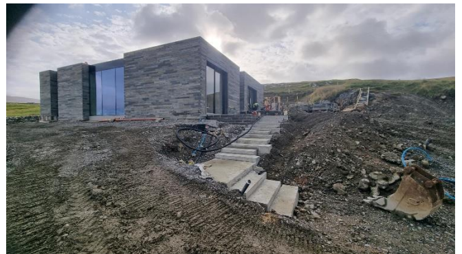
Parapet with concealed roof of neighbouring Dualchas Architects project in Sgarasta Mhor
