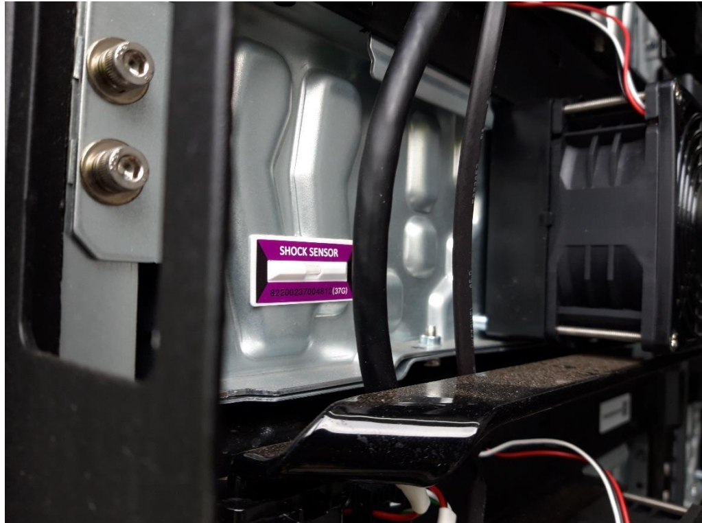
Figure 5. Shock Sensor Device Fitted to Battery Unit at Greenspan Energy Battery Project.
