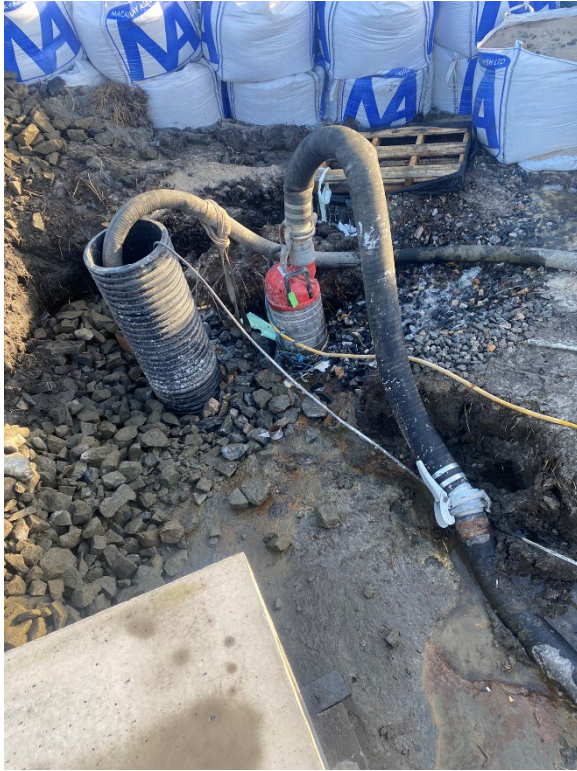
Photo 7 Pump heads and cowl system
