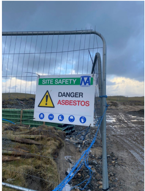
Photo 4 Asbestos warning signage and fencing
