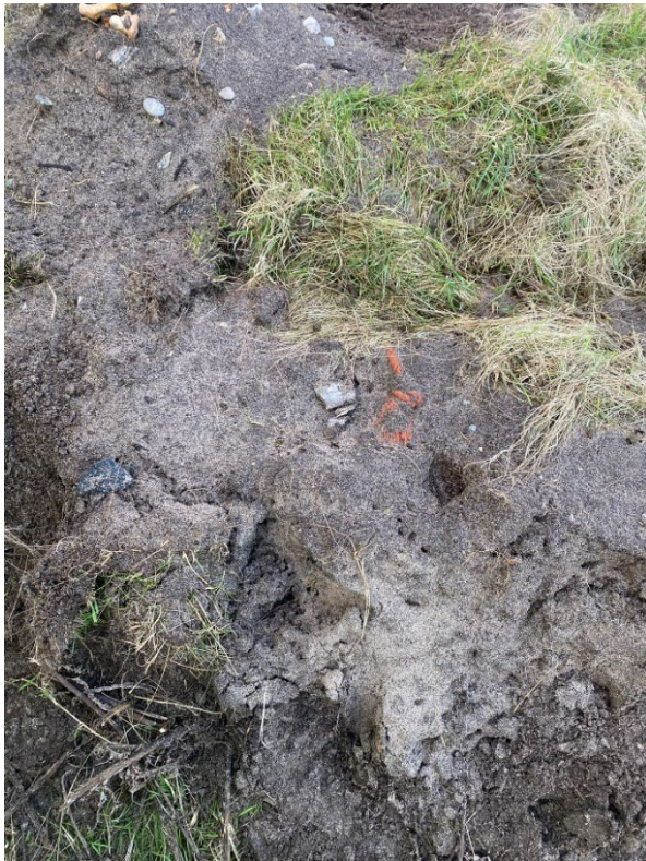
Photo 3 Asbestos in arising behind Byre 3
