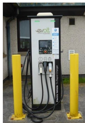
Figure 19 EV charging point
