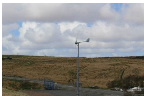
Figure 2 Evance turbine and housing site.
